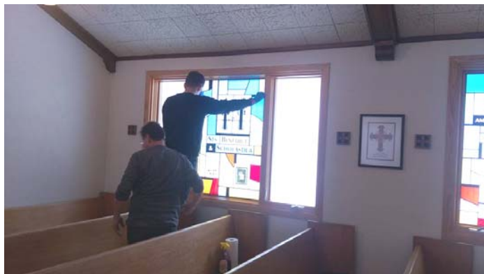
Michael Orchard and Nick Walberg from Michael Orchard Studio install the Sts. Benedict and Scholastica window.
